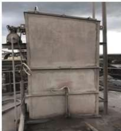
Fly Ash Silo De dusting Bag Filter
