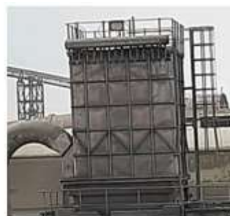
Coal Transfer point Bag filter
