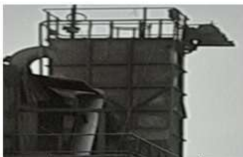
Coal hopper De Dusting Bag filter
