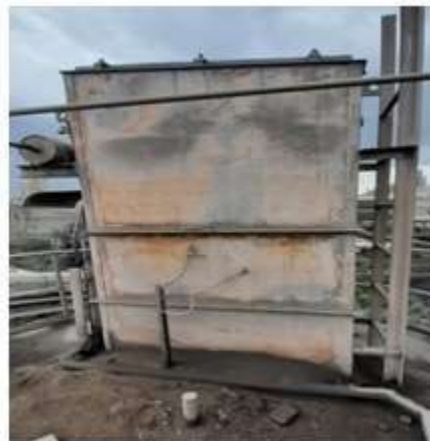
Bed Ash Silo Bag Filter
