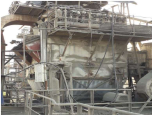
Coal Mill Venting Bag Filter
