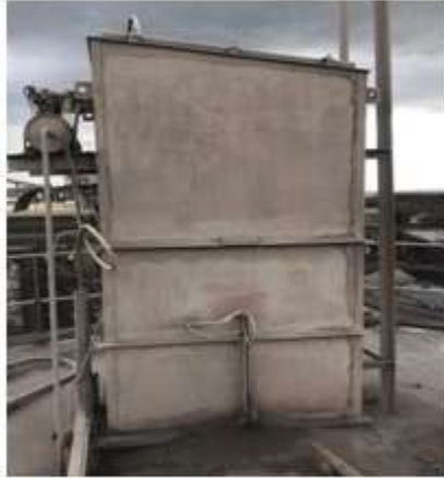
Fly Ash Silo De dusting Bag Filter
