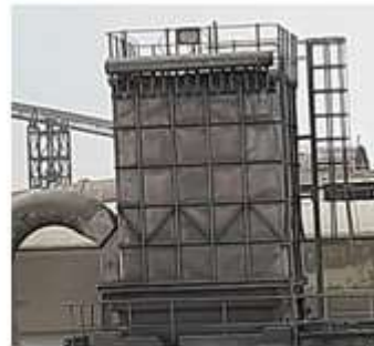
Coal Transfer point Bag filter
