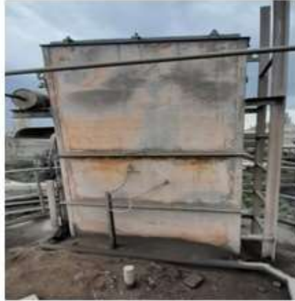
Bed Ash Silo Bag Filter
