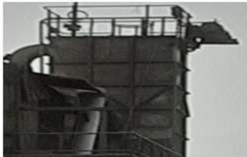
Coal hopper De Dusting Bag filter
