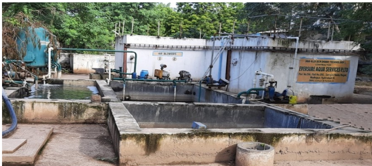
Sewage Water Treatment Plant for Domestic Water Treatment.
