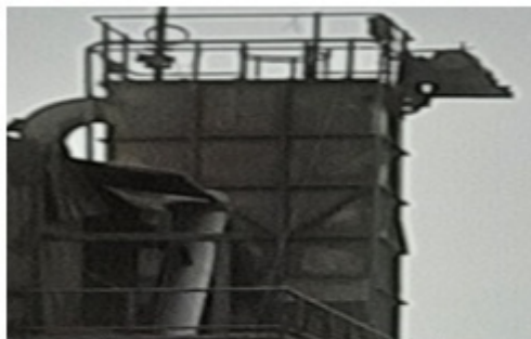
Coal hopper De Dusting Bag filter
