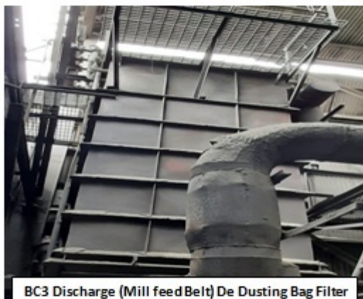
BC3 Discharge (Mill feed Belt) De Dusting Bag Filter
