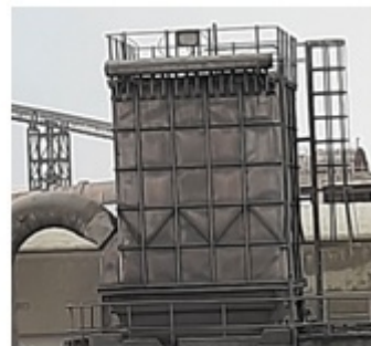
Coal Transfer point Bag filter
