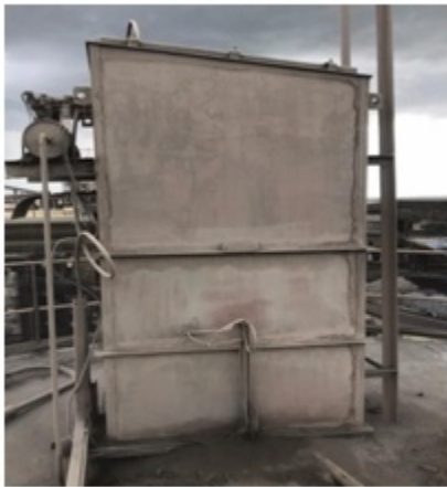
Fly Ash Silo De dusting Bag Filter
