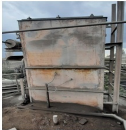
Bed Ash Silo Bag Filter
